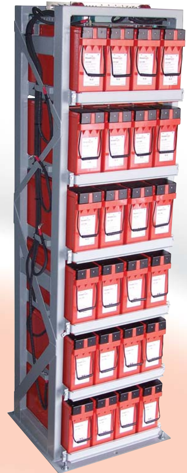
48V 1,140Ah System Six Strings of SBS190F
